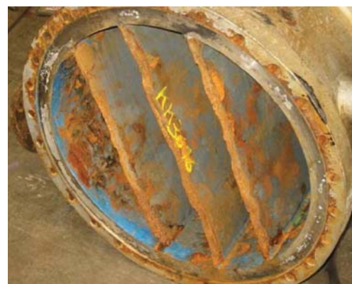
5 year old steel coated channel (credit TOTAL).
