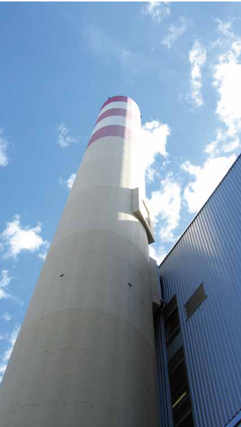
KOREMA® expansion joint on stack of waste fuelled power station
